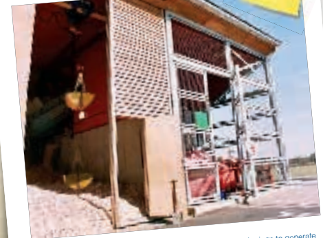
The "combined heat and power" plant at BedZED uses tree clippings to generate electricity and provide hot water to residents.
