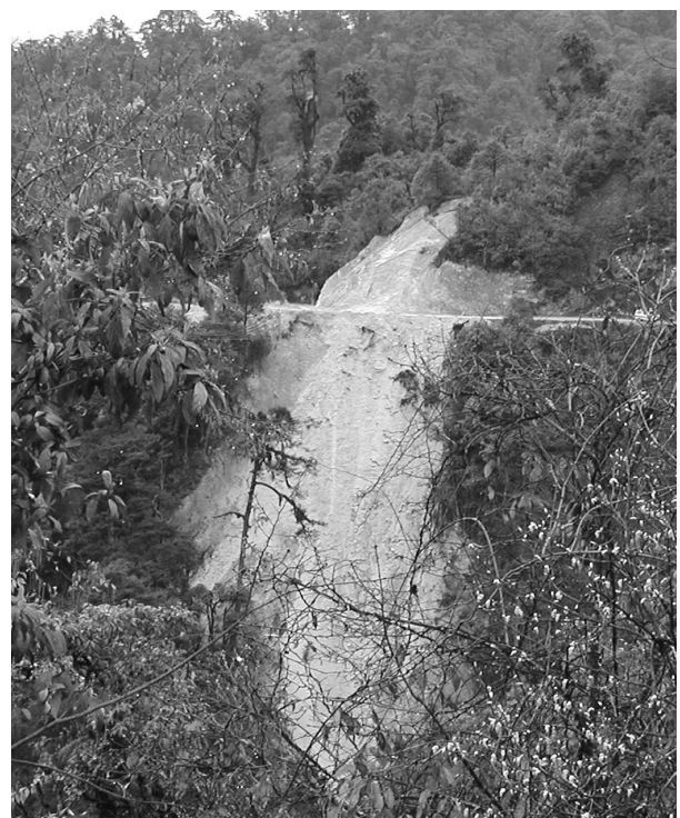
Erosion from road construction
